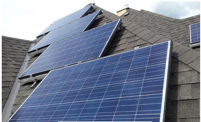
Figure 6: Roof-mounted Solar PV
