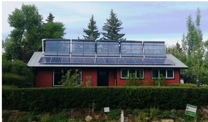
Photo of solar PV modules and solar thermal collectors
