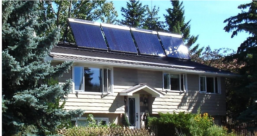
Figure 4: Solar Thermal Collectors
