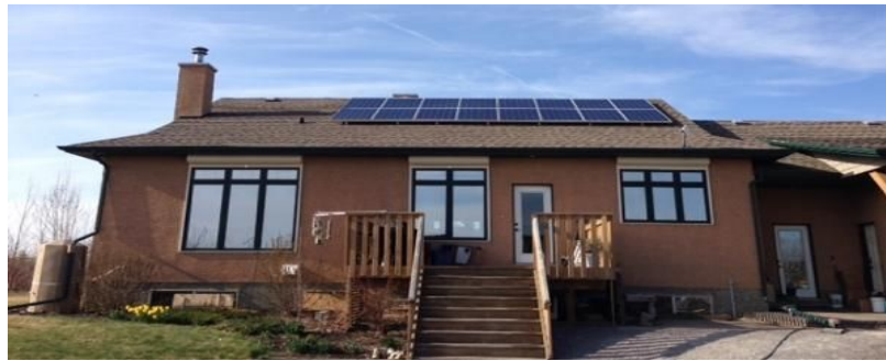
Figure 2: Solar PV Modules
